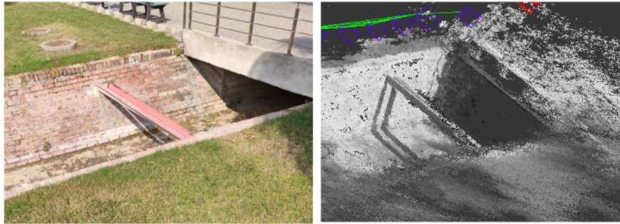
Figure 5-8: Left : Image showing a bridge and an associated pipe structure over a waterway. Right : Shows the reconstruction of a bridge and pipe structure in a 3D point cloud for inspection.
