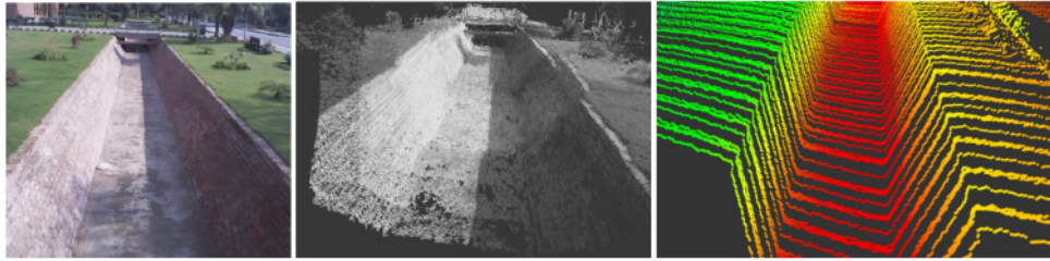
Figure 5-6: Left : An RGB image representing a section of a real water canal during a test flight. Middle : Shows a 3D point cloud of the same waterway section, generated using Visual trajectory only. Right : Shows a detailed map in point cloud generated by BottomLiDAR using a fused trajectory by our proposed EKF approach.
